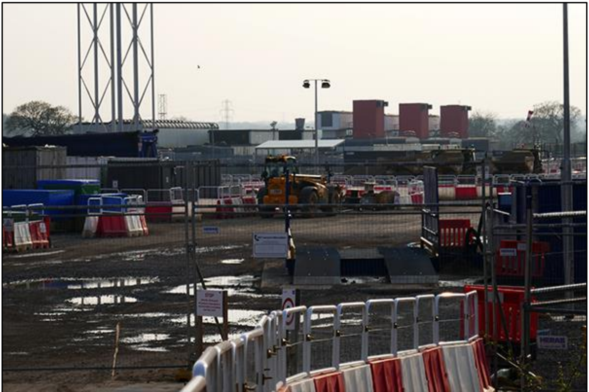
National Grid gas compressor station
